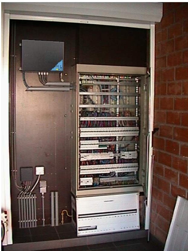
Figure 2: Clear division between input and output cables
