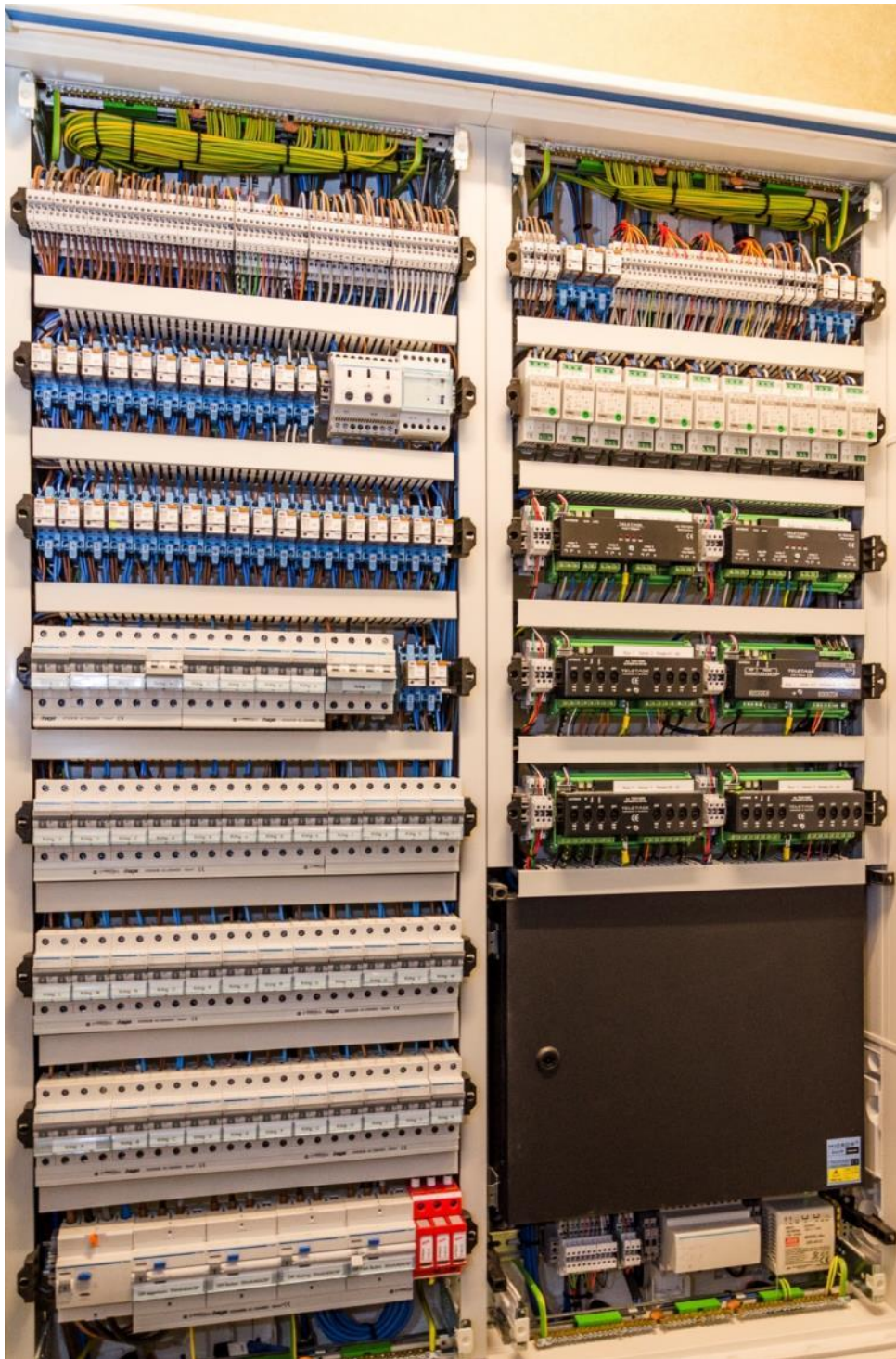
To protect the electrical installation and all equipment in the house, the distribution board is provided with over-Voltage protection (red block)
